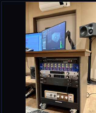
RACK - SALA DE CONTROL
